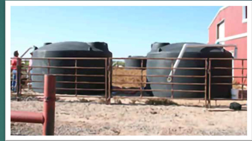
Storage tanks with an overflow pipe
