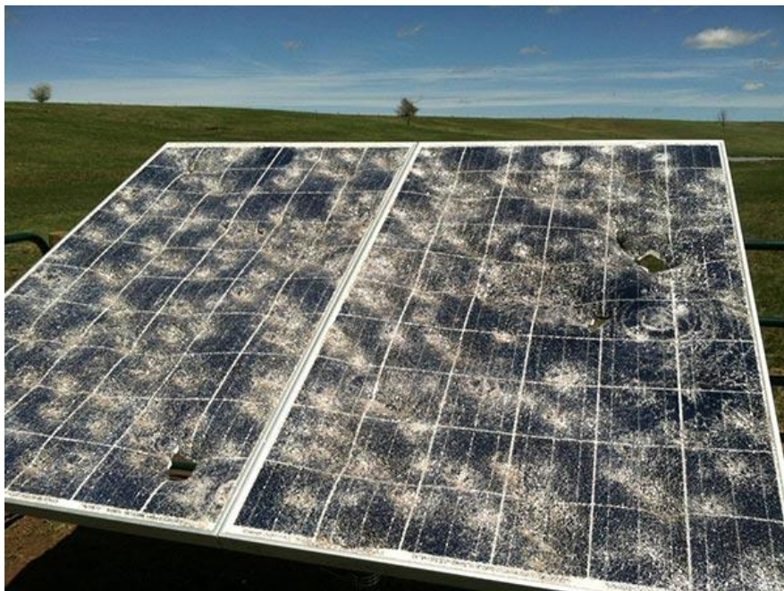
Damaged solar panel due to hail in south central Nebraska.. Photo courtesy of Tyler Williams, University of Nebraska
